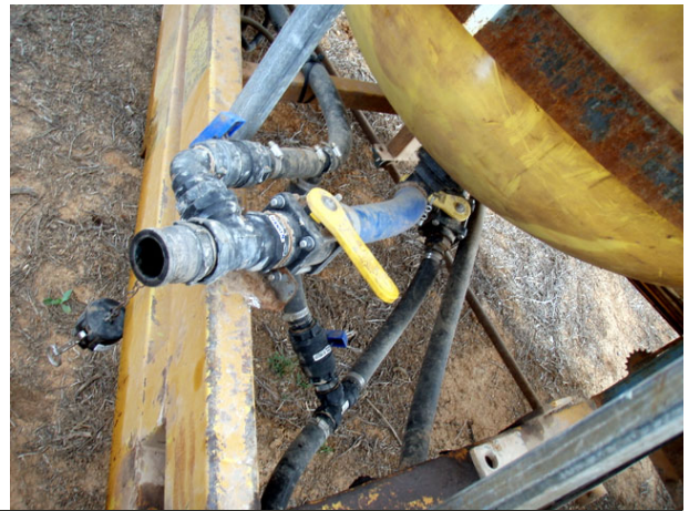
Above: 2 inch Cam lock fill point with taps to fill either main or flushing tank.
