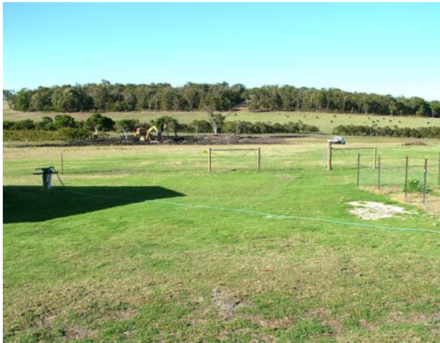
23 rd Feb 2005. Had a bit of rain. One of two new dams being built in Paddock 1 (in middle), Paddock 5 back right, neighbours back left.
